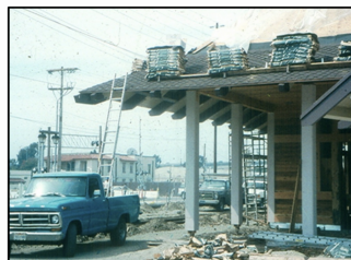
Can you identify any ladder violations or hazards in this picture?
